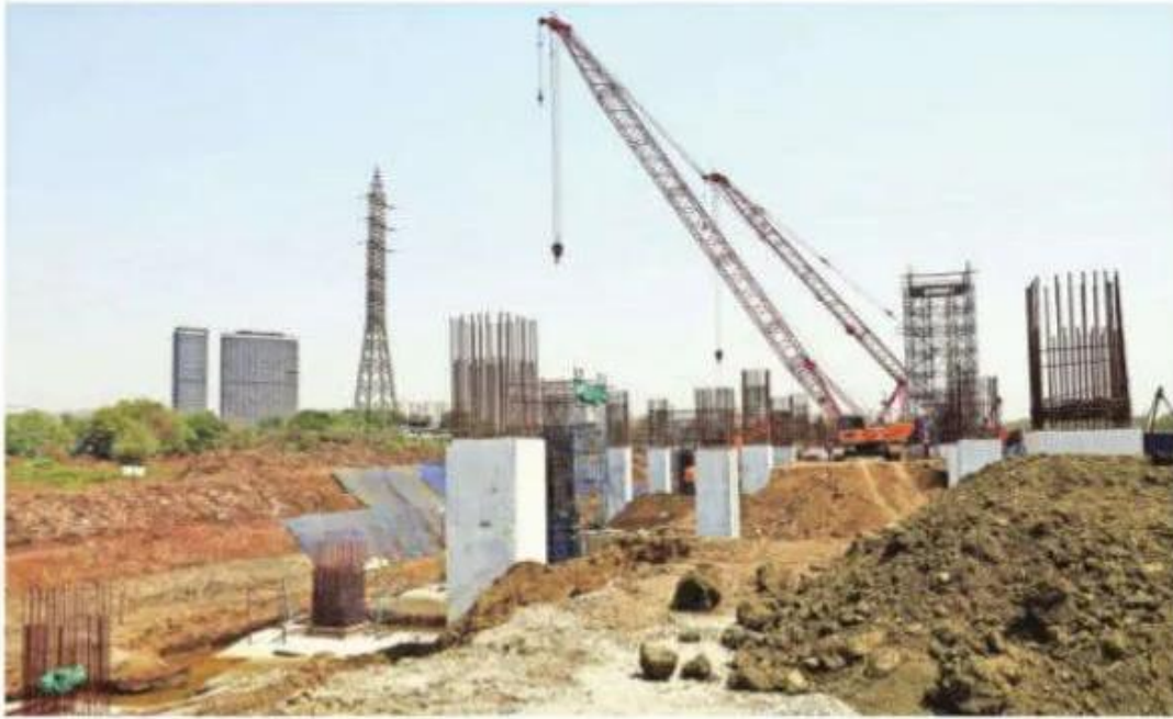
Construction of the Mumbai-Ahmedabad bullet train line underway at a Thane village. Deepak Joshi
